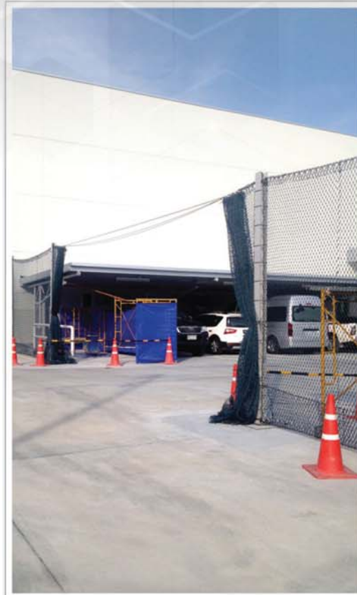
NET FENCE & SLIDE GATE
